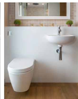
Residential: Installed at Mulberry House
