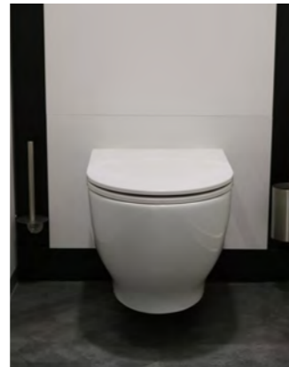
Commercial: Installed at Mettler Toledo Safeline
