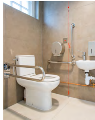
Leisure: Installed at Dover Castle
