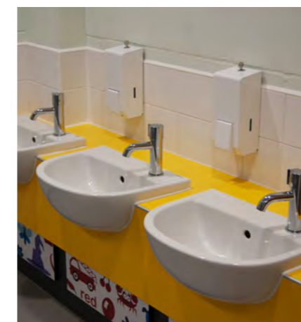
Installed at: Cottenham Nursery
