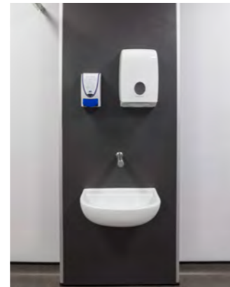
Healthcare: Installed at Acre Mills Hospital
