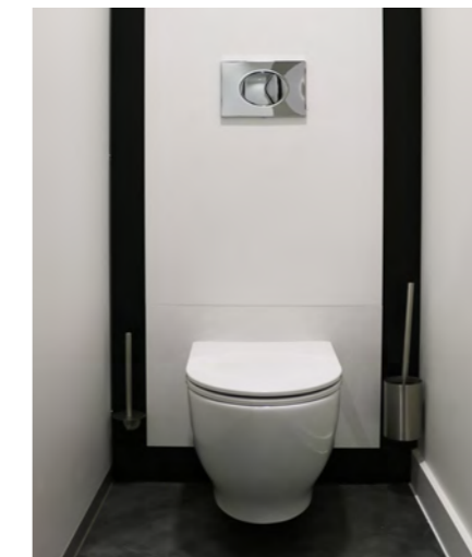
Installed at: Mettler Toledo Safeline
