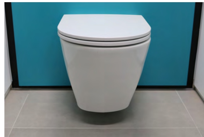
Commercial: Installed at a Richmond Magistrates Court
